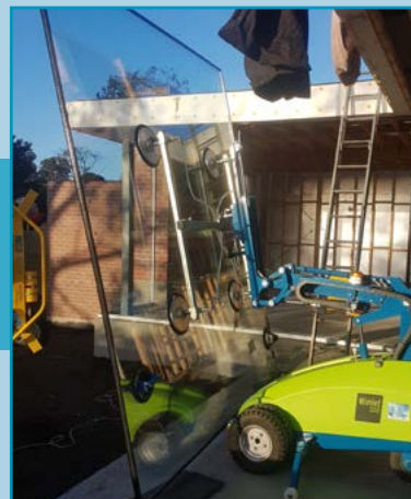
A Winlet 350 being craned onto site and then Installing double glazed units.
